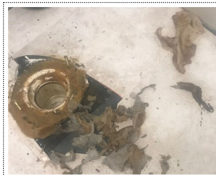
Homeowner Toilet Base
