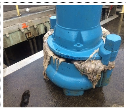
Wastewater Machinery Blockage
